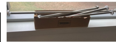
Vacuum spools leak tested
